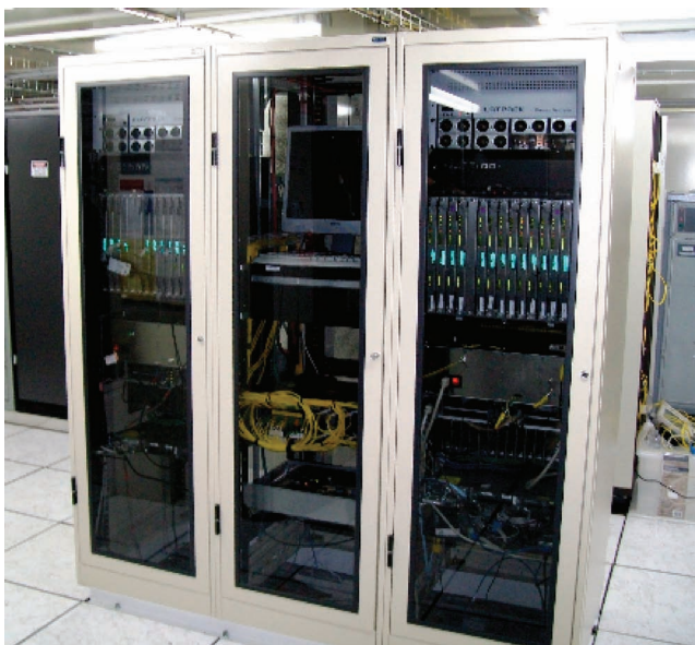
Figure 14. The CABB rack as installed in the fully shielded ATCA correlator room.
