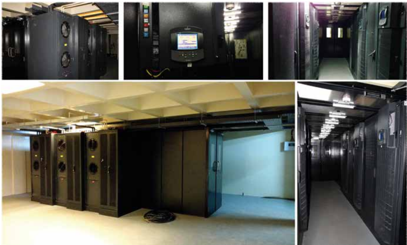
Figure 1. The data centre, a modular system, with the server racks, high density cooling systems and cold aisle containment.
