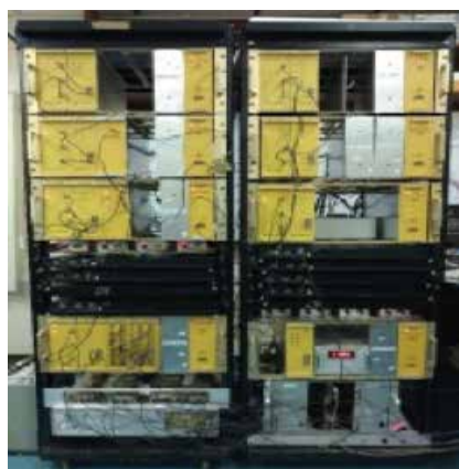
Figure 9. Racks housing the receiver systems.
