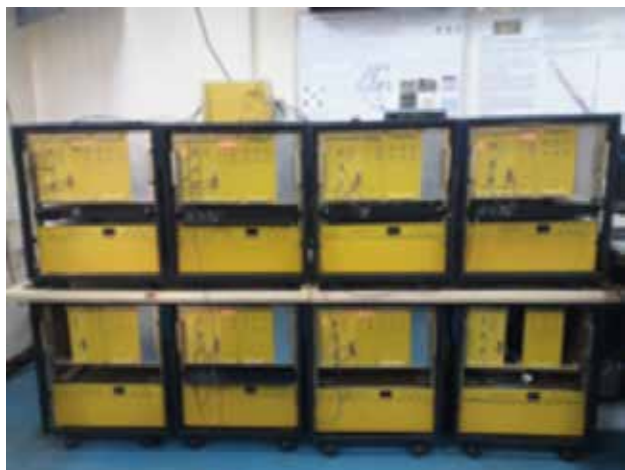
Figure 6. Hardware units, rewired and ready for future relocation to different Institutes
